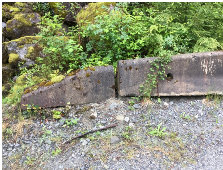
Bullnoses not attached at right approach
