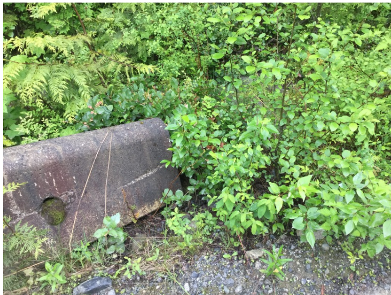
Missing bull nose at upstream left approach
