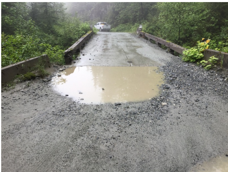
Large pothole at left approach
